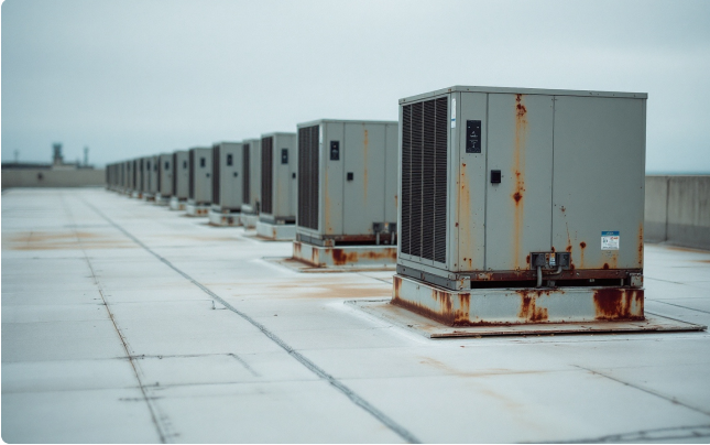
Photo 14, ref M-1. Rooftop units 1 through 4, original to building. Cabinet corrosion at base rails and coil sections. View north.
