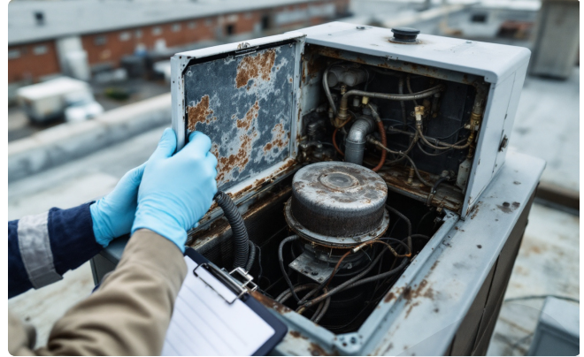
Photo 17, ref M-1. Unit 3 service panel open. Condenser coil fins deteriorated, compressor failed on test.
